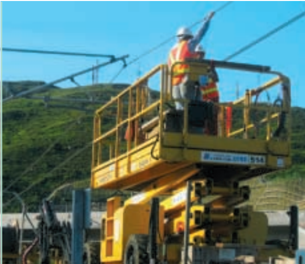
Installation of contact wire for the Overhead Line System on MTR Corporation's new Penny's Bay Line.
