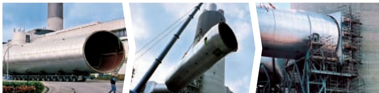
Transporting, lifting and installing an exhaust duct at Black Point Power Station
