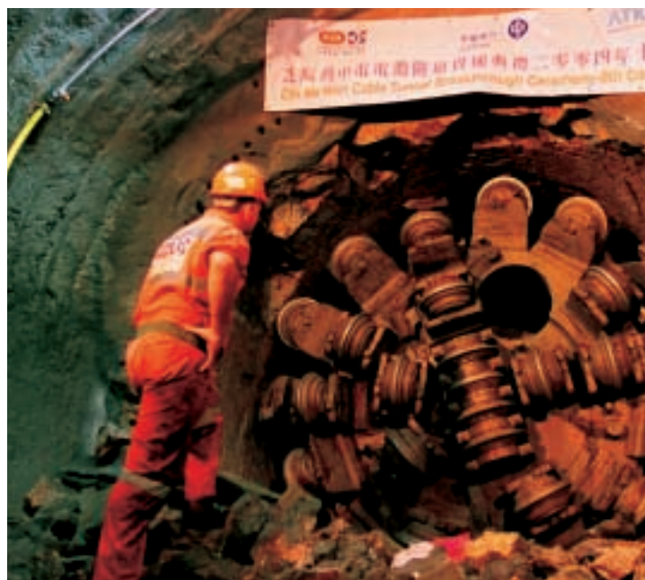
Breakthrough at the Chi Ma Wan Tunnel on the South Lantau to Cheung Chau 132kV cable project
