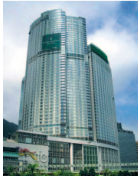
Installation of lifts and escalators and curtain walls for Four Seasons Hotel at Hong Kong Station Development
