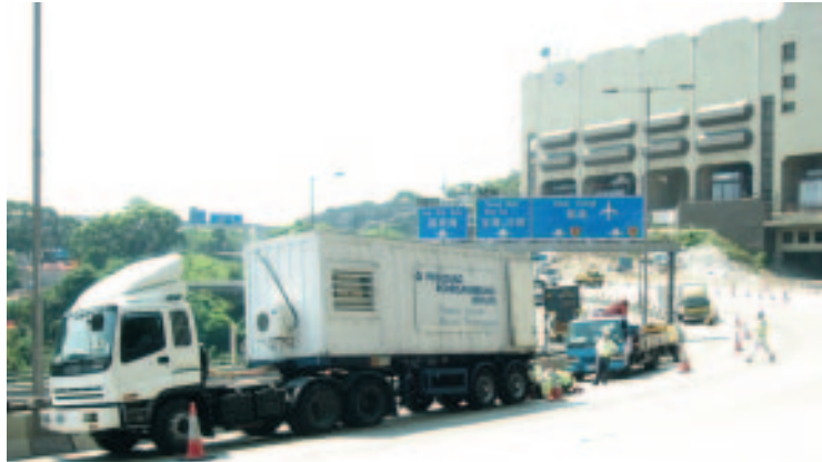
Relining of DN750 Storm Water Drain by Process Phoenix at Ching Cheung Road
