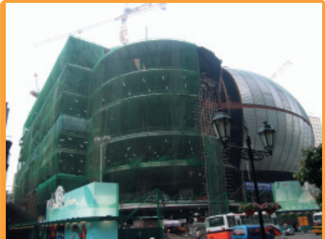
Installation of HVAC system for Grand Lisboa Hotel in Macau, which is under construction
