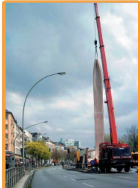
Pipe rehabilitation projects of Chevalier exist all over the world. Picture shows the project at Hamburg, Germany
