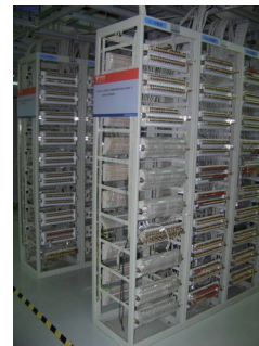
Digital distribution frame
