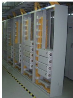
Optical distribution frame
