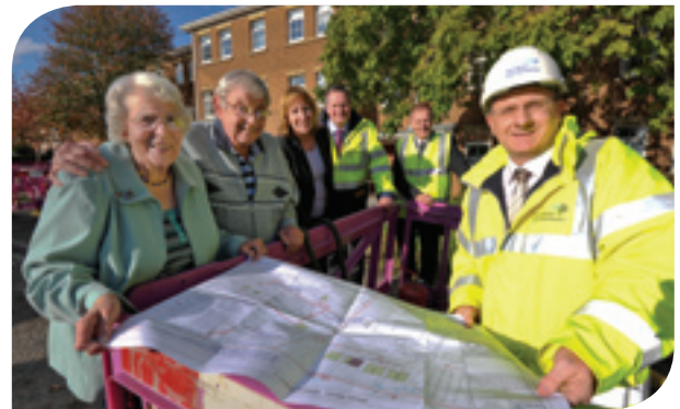
NGN helps combat fuel poverty in the local community with the extension of gas supply network and installation of new energy efficient central heating systems.
