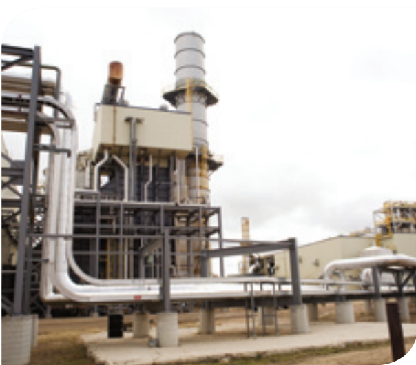
The Meridian power plant notches the best scores in safety and environmental performance.
