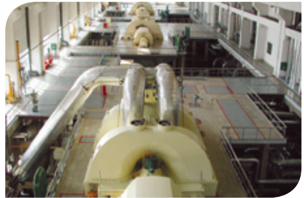
We strive to achieve world-class performance in electricity and heat generation.
