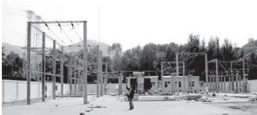
Figure 12-1: Newly Built 35 KV Gemengou Substation
