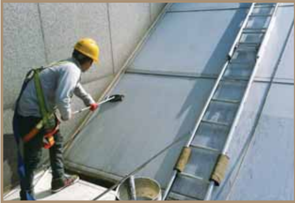
Training on Use of Fall Arrestor System
