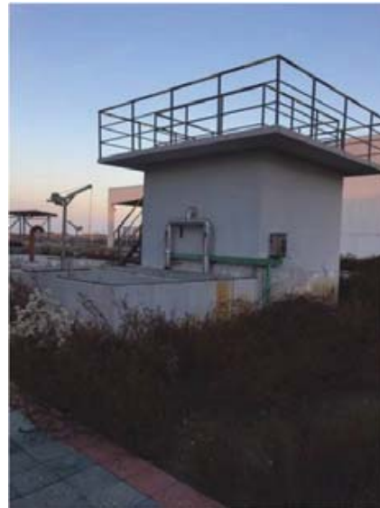
Sewage Station – Sludge Tank
