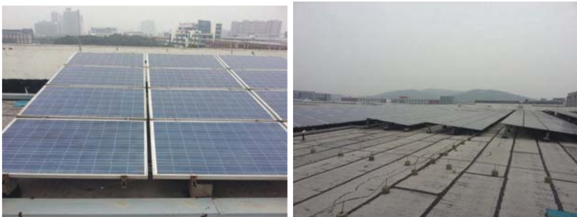
Figure 6.4 Photovoltaic (PV) Module Arrays
