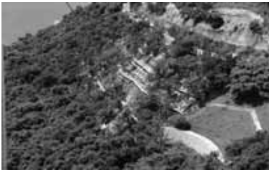
Installation of soil nails, erosion control mat and wire mesh, maintenance stairway
