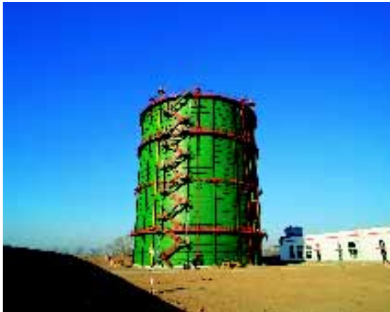
Cylinder-shaped gas storage tank in Langfang
