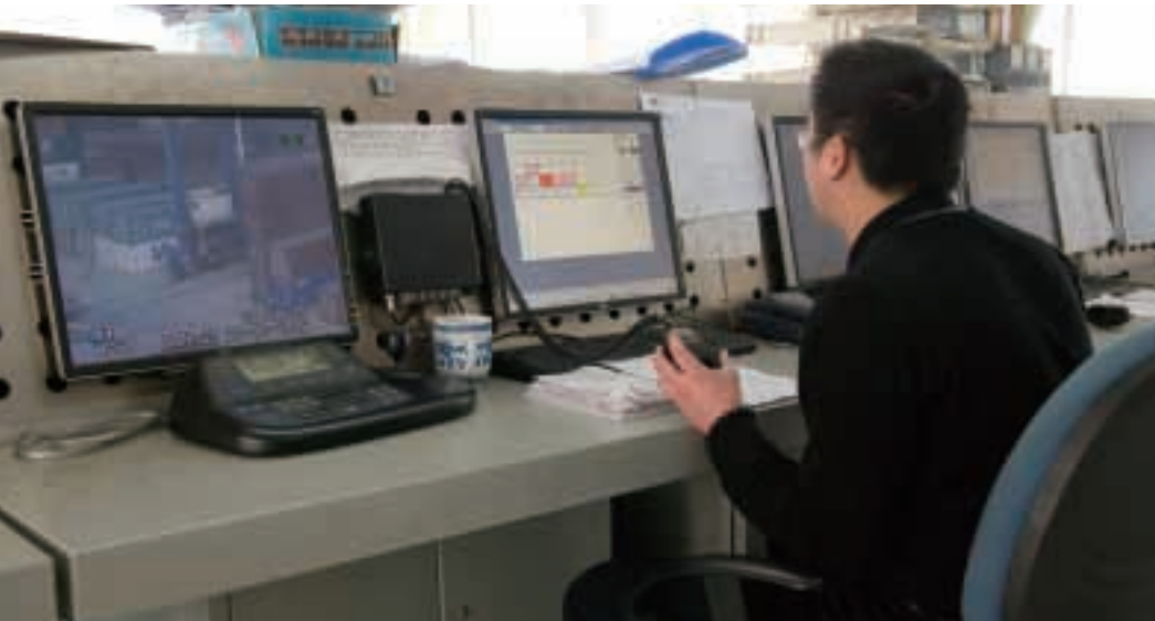
Computer Terminal Management System (CTMS)
