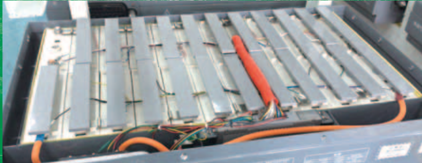
Battery Pack: Single integration of BMS cells
