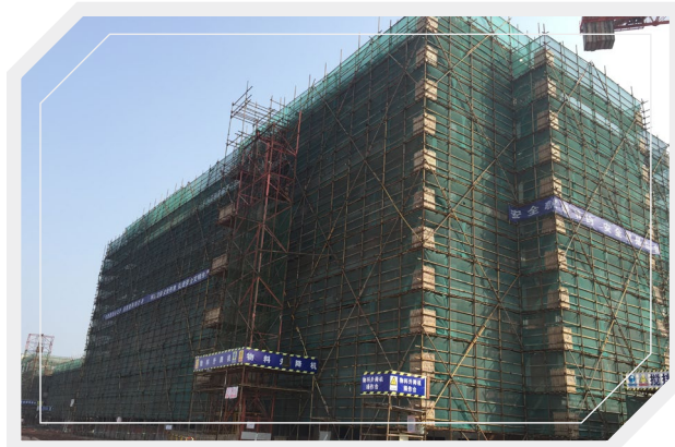
The administrative building of Zhejiang Forever New Energy Limited is approaching completion
