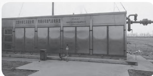
On-site photo of the oil vapor recovery unit of Zhongnanhui 圖：中南匯油氣回收裝置現場照片
