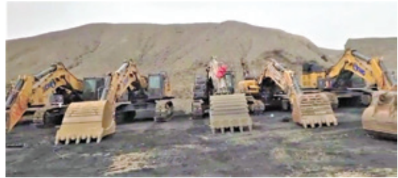
The coal fire extinguishment project will be carried out in the form of stripping and leveling
