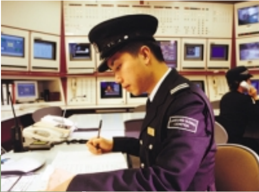
Top security is ensured at all times with 24 hour monitored security CCTV system at Cheung Kong Center.
