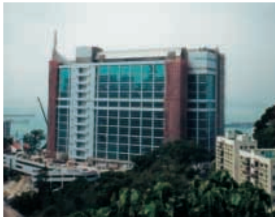
Project of the New Medical Complex at the University of Hong Kong
