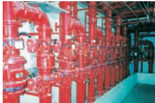
Fire Services Sprinkler Control Room
