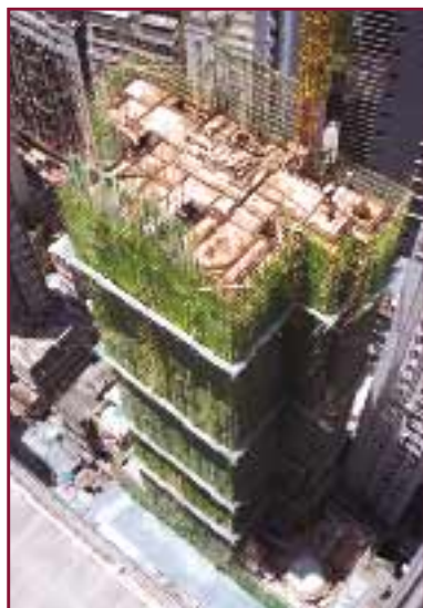
Superstructure construction for The Grandeur and Grandeur Place at 44 Jardine's Crescent & 47 Jardine's Bazaar, Causeway Bay, Hong Kong
