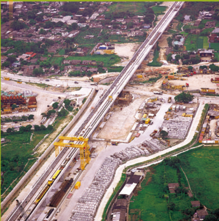
West Rail Phase 1 – Construction of viaduct from Tin Shui Wai to Tuen Mun North
