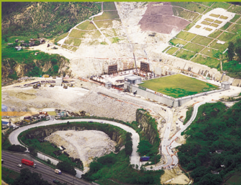
Construction of Tan Kwai Tsuen North Fresh Water Service Reservoir, Yuen Long
