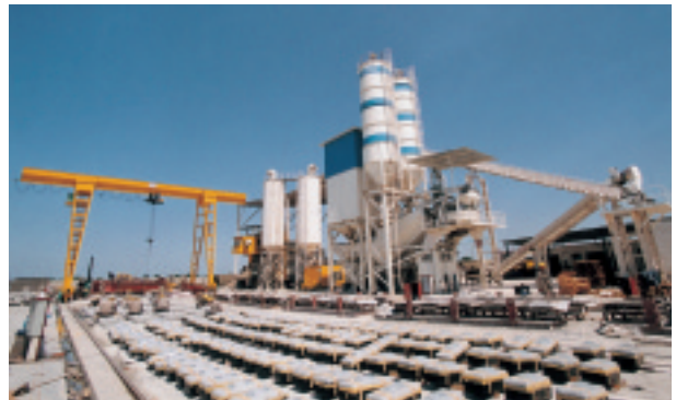
Precast concrete products factory in Dongguan, PRC
