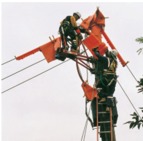
In general, overhead line repair and maintenance work requires the power to be shut off, causing disruption to the electricity supply. With a view to minimising such interruptions, a team of highly skilled staff is carrying out live line maintenance work which is a technology introduced in CLP Power in 1999.
