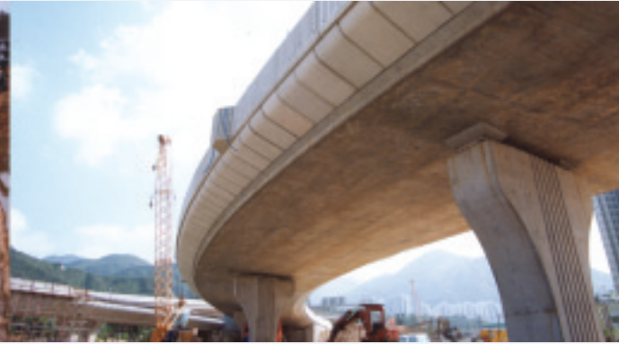
Ma On Shan Development Phase 3 (Completion Contract for Contract S) – Formation, Roads, and Drains in Areas 77 and 86
