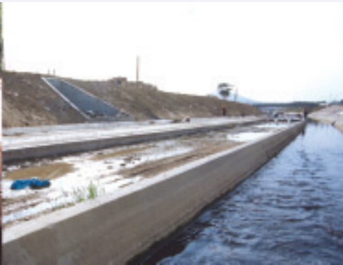
Construction of Main Drainage Channels for Yuen Long and Kam Tin Stage II – Kam Tin San Tsuen to Wang Toi Shan Section
