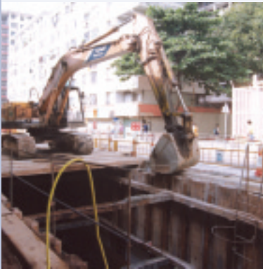
North West Kowloon Sewerage Stage III Phase II and West Kowloon Storm Water Drainage Improvement Stage I Lai Chi Kok, Cheung Sha Wan & Sham Shui Po Areas
