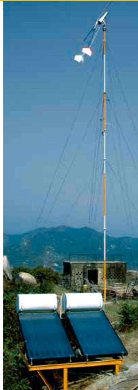
Hybrid solar-wind renewable energy system in Shek Kwu Chau, Hong Kong
