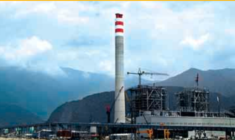
Ho-Ping Power Station, Taiwan
