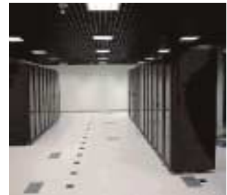
Hosting services delivered through data centres
