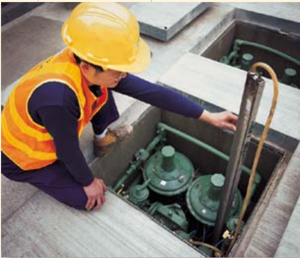
A regular maintenance check on one of our newly-designed underground gas governors.
