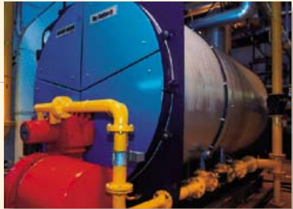
High-performance gas steam boilers are now in service at Queen Elizabeth Hospital.
