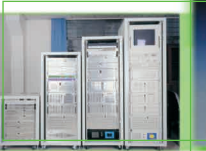
IPC Server Cabinet (IPC-9000 A.B.C.D.)
