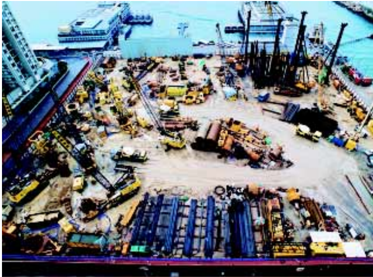
Bored piling and H-piling work at Inland Lot No. 8955, Sai Wan Ho, Hong Kong undertaken by Kin Wing Foundations Limited
