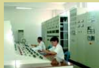
Power Station Control Panel
