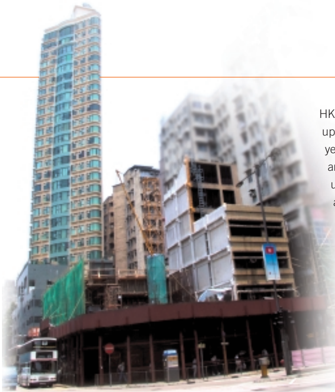
Front — Bijou Court II under construction, Behind — Bijou Court I at Prince Edward Road
