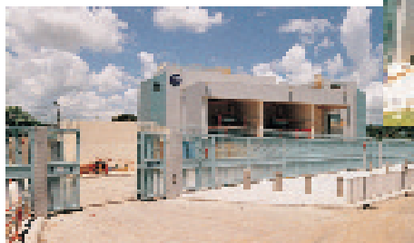
Tai Tao Tsuen Substation
