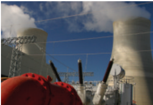
Mt. Piper Power Station electrical contracting and maintenance
