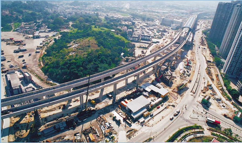
West Rail Phase 1 — Construction of viaduct from Kam Tin to Tin Shui Wai
