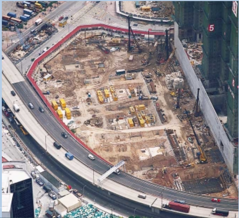
Foundation Works for the Proposed Residential Development at NKIL 6275 West Kowloon Reclamation
