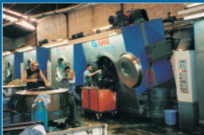
Industrial washers and centrifugal separators in washing room located in Guatemala.
