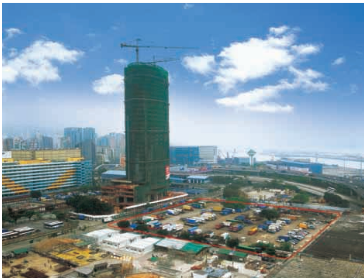
The construction of Enterprise Square 3 in progress with the site of Enterprise Square 5 in the foreground outlined in red in Kowloon Bay
