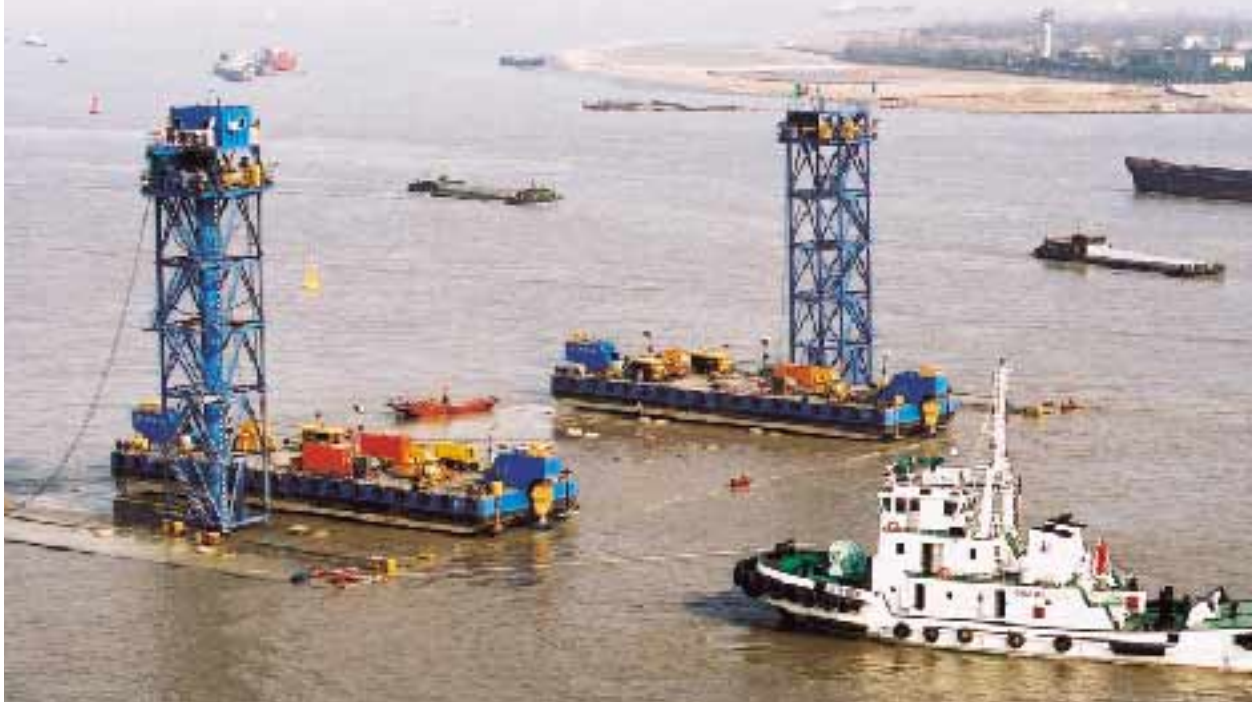
Marine Works-Towing and Sinking Preparation of Element 沉埋管的拖運及沉放準備工作
