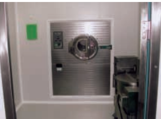
Newly-acquired facility: High efficiency thin sugar-coating machine
