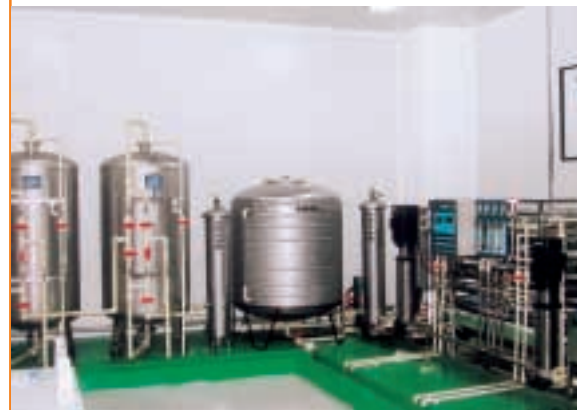
Newly-acquired facility: Pharmaceutical purified water treatment system
