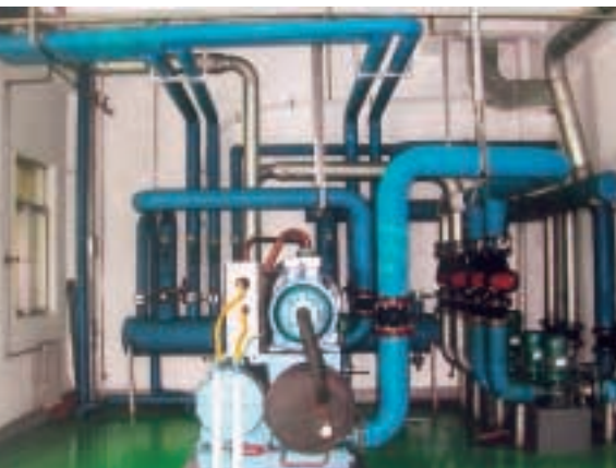
Newly-acquired facility: Pharmaceutical workshop refrigeration system
