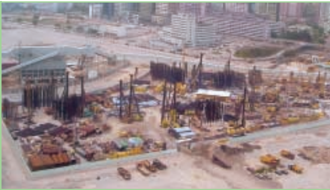
Bored piling and H-piling work at South East Kowloon Development Site 1A-Phase 1 at North Apron Kai Tak Airport, Kowloon, undertaken by Kin Wing Engineering Company Limited
