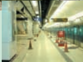
Supply and Installation of Structured Cabling System and Fibre Network in Metropolitan Area Network (MAN) for nine stations, maintenance centre and West Rail Building of KCRC West Rail
