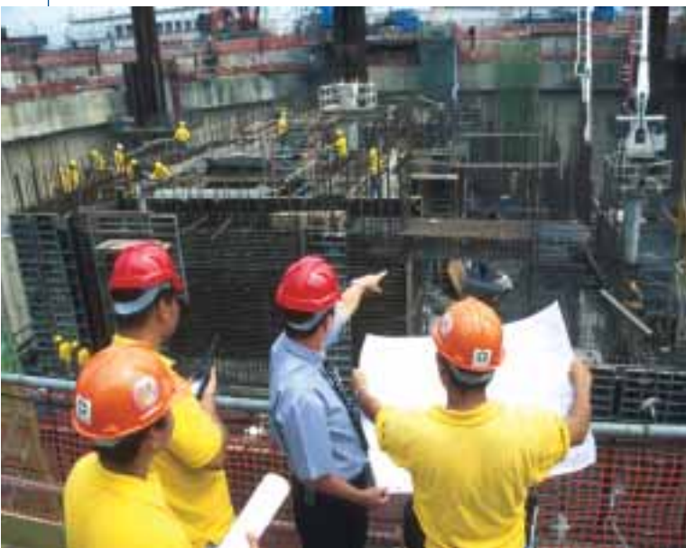
Superior management and vertical integration allow the Group to maintain premium quality of its developments while reducing construction costs.
