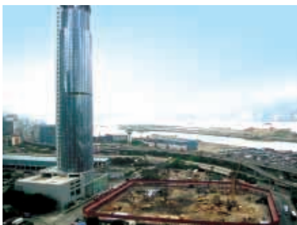
The construction of Enterprise Square 3 in progress with the site of Enterprise Square 5 in the foreground in Kowloon Bay
