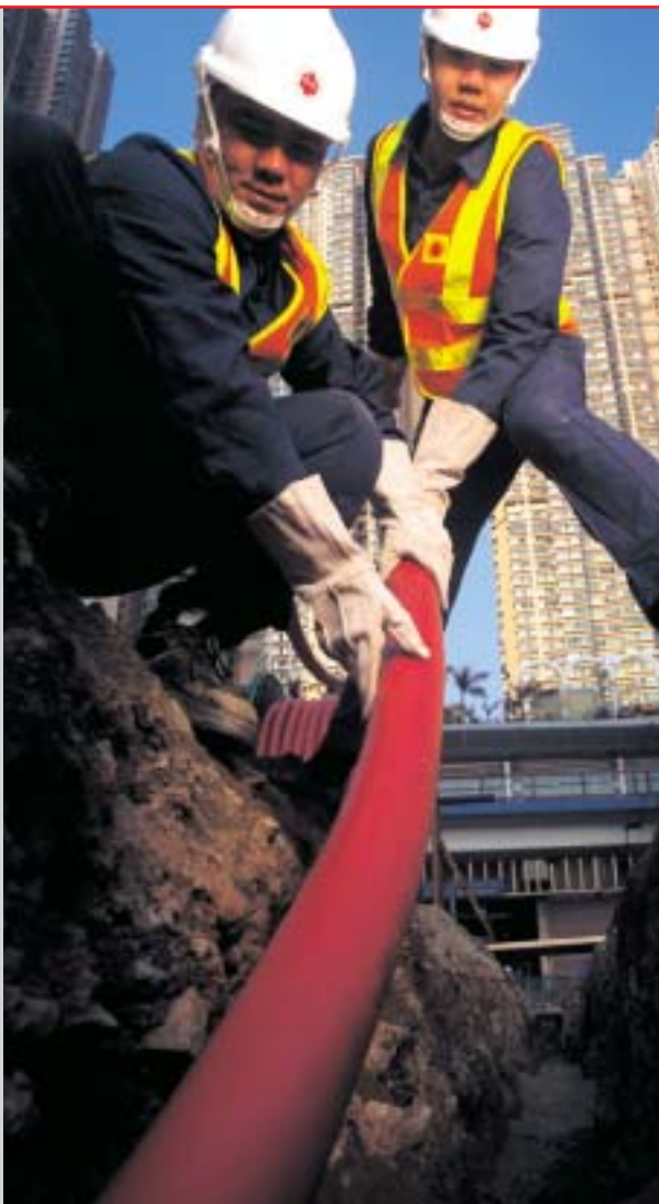
New cable, the lifeline of our transmission network being laid as part of a continuous effort to reinforce the system and cater for new demand.
