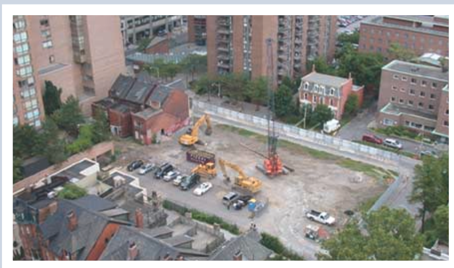
Commencement of construction of One St. Thomas Residences, Canada's most luxurious residential building designed by Robert A.M. Stern.
