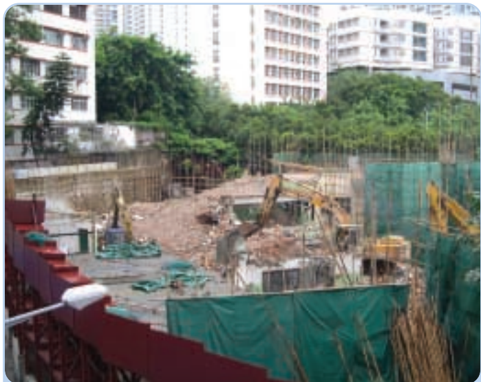
Demolition works at 97 Po Kong Village Road, Diamond Hill, Kowloon in progress
