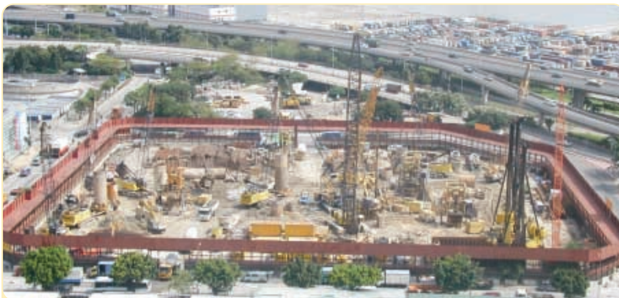
Bored piling works for Enterprise Square 5 at New Kowloon Inland Lot No. 5927, Kowloon Bay, Kowloon
