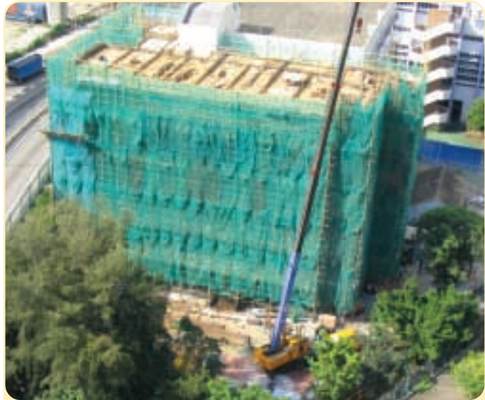
Superstructure works of Lai King Catholic Secondary School at Lai King Estate, Kwai Chung, New Territories
