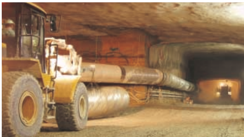
Underground excavation for Lane Cove Tunnel commenced in April 2004 and steady progress is being made.
