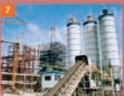
7 Yushe Power Plant (800MW)
