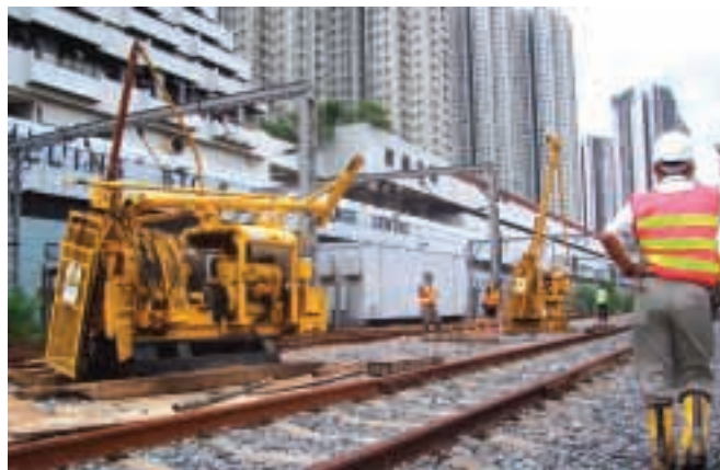
Pre-drilling works for KCRC Ho Tung Lau (Site A) Development undertaken by DrillTech Ground Engineering Limited
