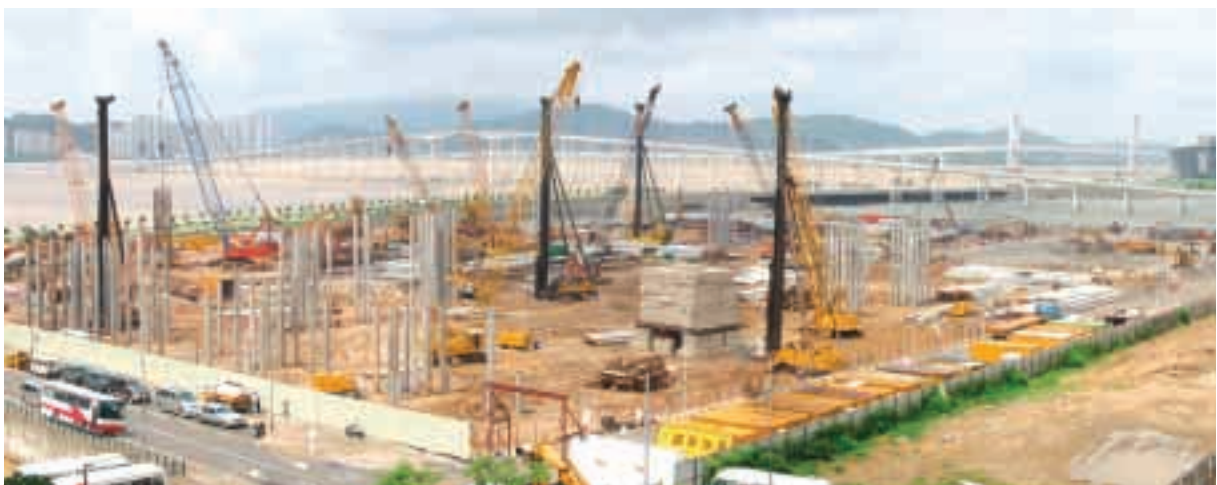
Daido piles and sheet piles at MGM Grand Macau at Nam Van, Macau undertaken by Chinney Timwill Construction (Macau) Co., Ltd. and Kinwing Engineering (Macau) Company Limited
