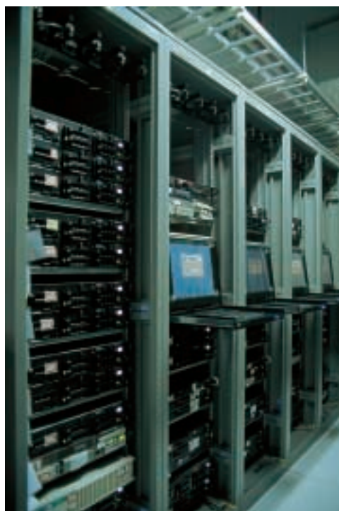
Hi-tech standard IDC room
